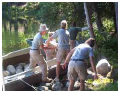
Using the "Rock Barge" to transport 45 tons of rock across Cobbossee Stream.
